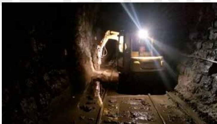
Picture 5. Prepared substrate excavations, new central drainage line and new sleepers and rails
