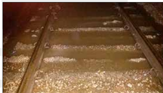
Picture 4. Detailed image of tracks condition at certain parts
