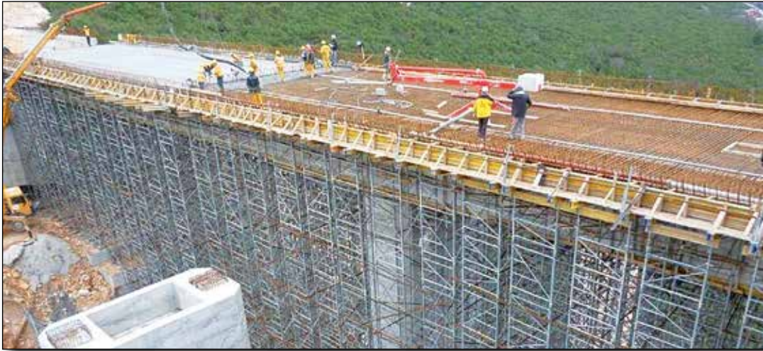
Figure 15. Concreting span structure S4D of Studenčica bridge using combined concrete transportation by pump truck and stationary concrete pump with concrete spreader
